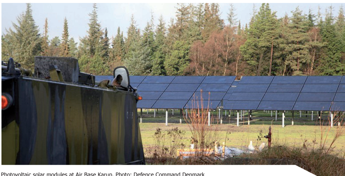
Photovoltaic solar modules at Air Base Karup. Photo: Defence Command Denmark
