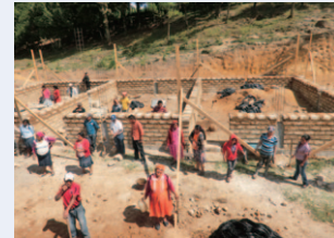
Additional classrooms are being constructed using local materials to enable children to study indoors in Yamaranguila Municipality, Intibuca Department. (Photo: FOCAL II Project)
