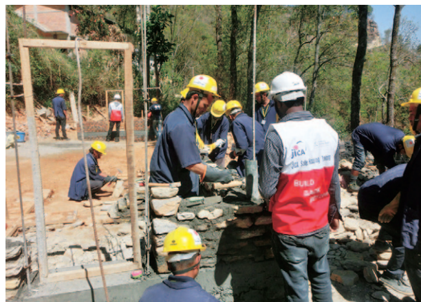
Architectural engineers receive residential construction training supervised and implemented by Japan in Chautara, Sindhupalchowk District in the eastern part of Nepal as part of the "Program for Rehabilitation and Recovery from Nepal Earthquake." (Photo: Kazutaka Isaka / JICA Nepal Office)
