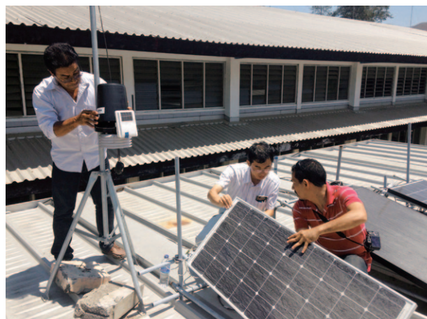
An expert, Dr. Nobukazu Kameyama (center) explains about the facility and equipment at a solar power generation facility to teachers of the Faculty of Engineering, Science and Technology at the National University of Timor-Leste on the outskirts of Dili. (Photo: Atsushi Takahashi)
