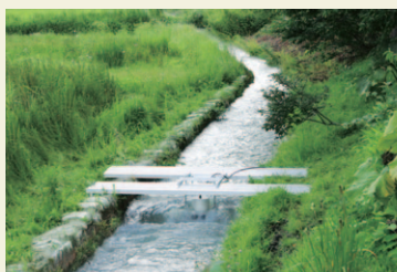
The “Cappa,” hydro-kinetic -power generator, in operation (Photo: ibasei)
