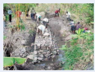
Weirs have been upgraded to masonry construction in the regions where irrigation farming with simple weirs is implemented successfully. (Photo: JICA)
