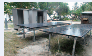
Ten solar-powered desalination plants (reverse osmosis membrane method) were installed on a remote island of Manus Province. They can desalinate sea water and purify ground water which clear the WHO drinking water standards in a location with absolutely no water or electrical infrastructure, and makes daily life possible without depending on uncertain and impure rain water. (Photo: Sojitz Corporation)
