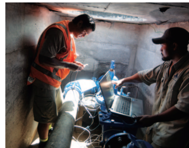
Flow volume management being carried out by the Samoa Water Authority Urban Section Non-Revenue Water Countermeasures Unit as part of the "Capacity Enhancement Project for Samoa Water Authority in Cooperation with Okinawa" (see page 155) (Photo: Kenta Tomiyama / JICA)
