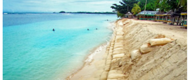
Resistant to punctures and ultraviolet rays, these sturdy, multiple-ply sand bags discreetly work double time as they protect the coastline and homes nearby. / C-CAP
