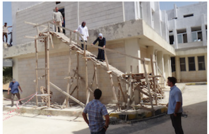
USAID Jordan Senior Civ-Mil Adviser Ben Kauffeld, CENTCOM Planner Haider Haider (not pictured), and members of incoming and outgoing CMSE teams, monitor second floor construction of the Kufranjah Health Center in Jordan. The clinic received assistance from USAID in 2014 and 2015, and CMSE Jordan provided assistance with clinic upgrades, expanding its capacity to Syrian refugees in Kufranjah. The upgrades are expected to be complete mid-December 2015. Photo credit: Ben Kauffeld
